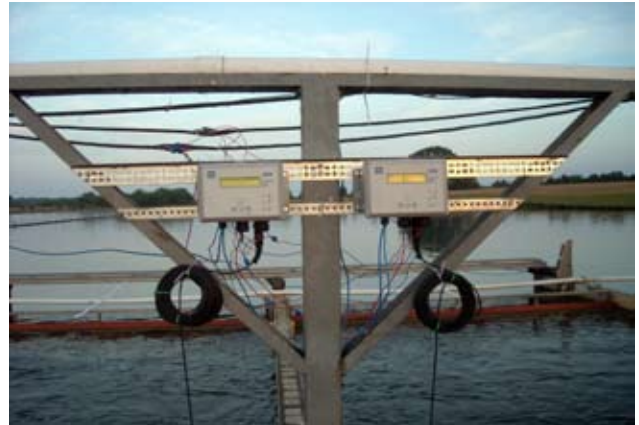
Each raceway is monitored with a YSI 5200 multiparameter monitoring and control instrument that tracks oxygen and temperature. The YSI 5200s activate oxygen blowers as needed; they will soon also be used to automatically deliver feed, adjusting for growing biomass. [Photo: Travis W. Brown]
